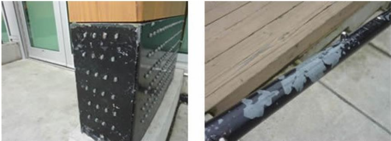
Chipping paint reveals neither primer nor surface preparation on underlying galvanized surfaces
