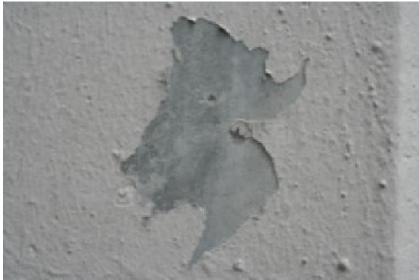
Concrete coating failure
