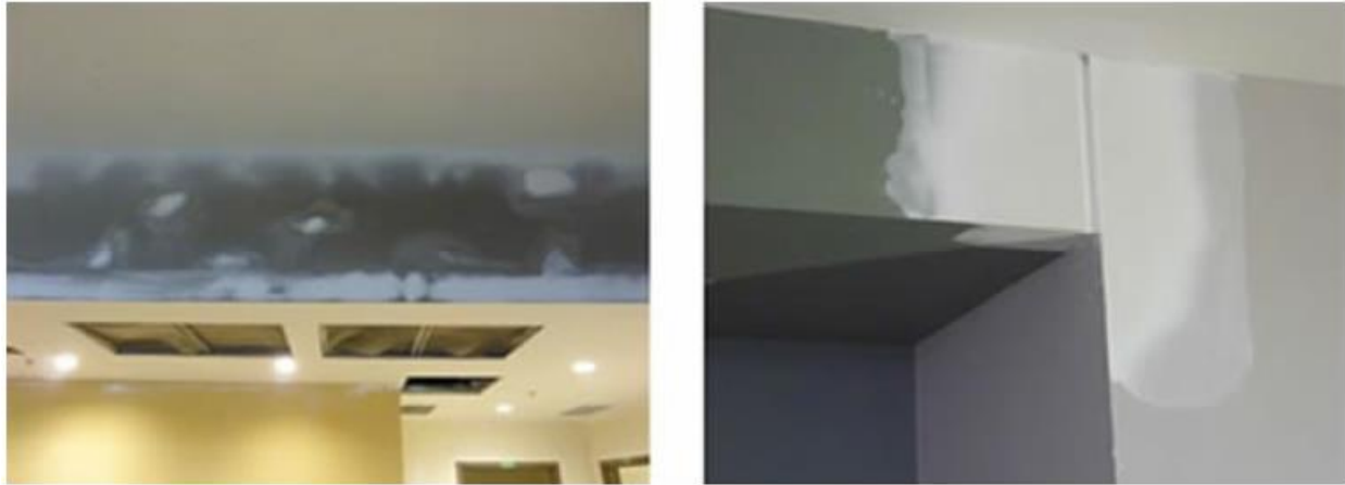
Excessive drywall repairs made after application of intermediate coat
